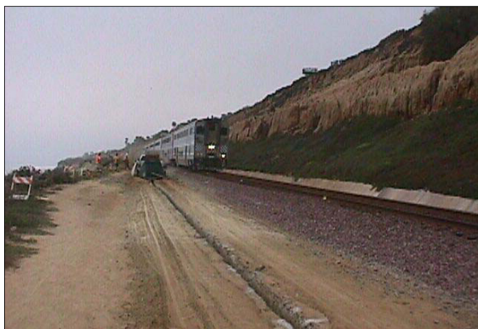
TDR Cables are buried parallel to the track and enclosed in a layer of concrete
